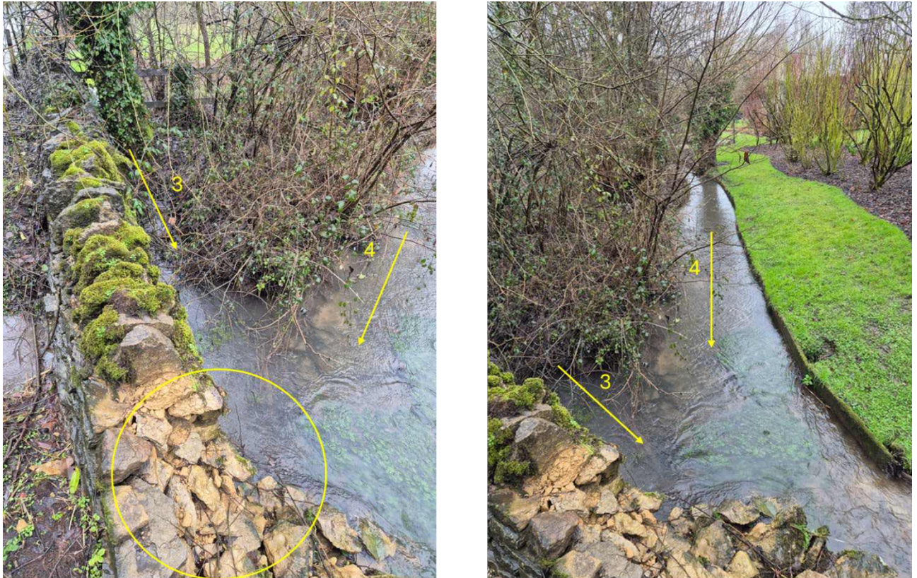
Figure 2-7 Confluence of watercourses 3 and 4 and observed damage to stone wall
