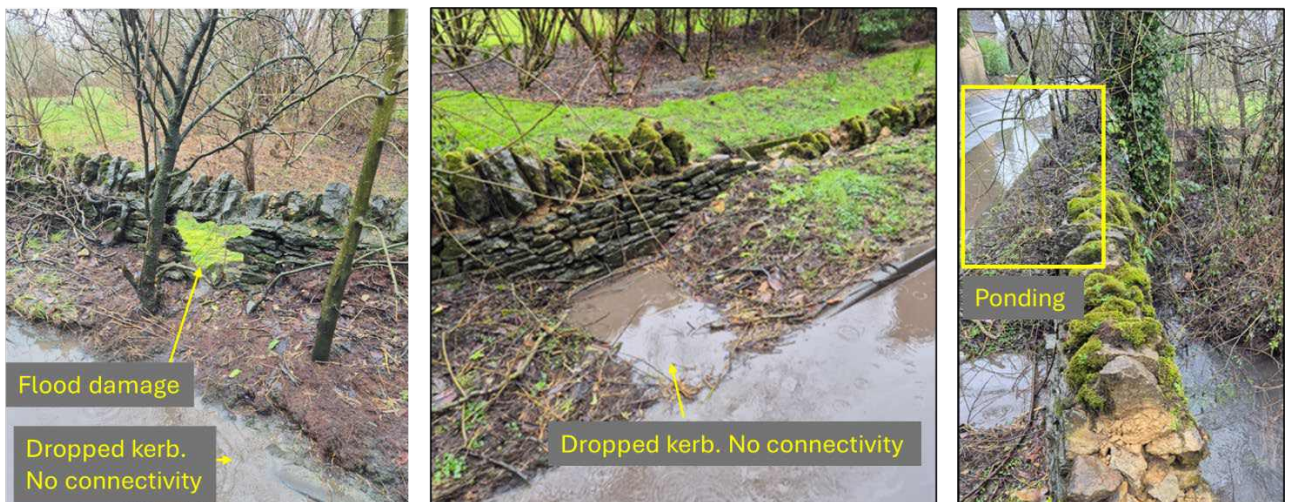
Figure 2-8 Highway Drainage Issues
