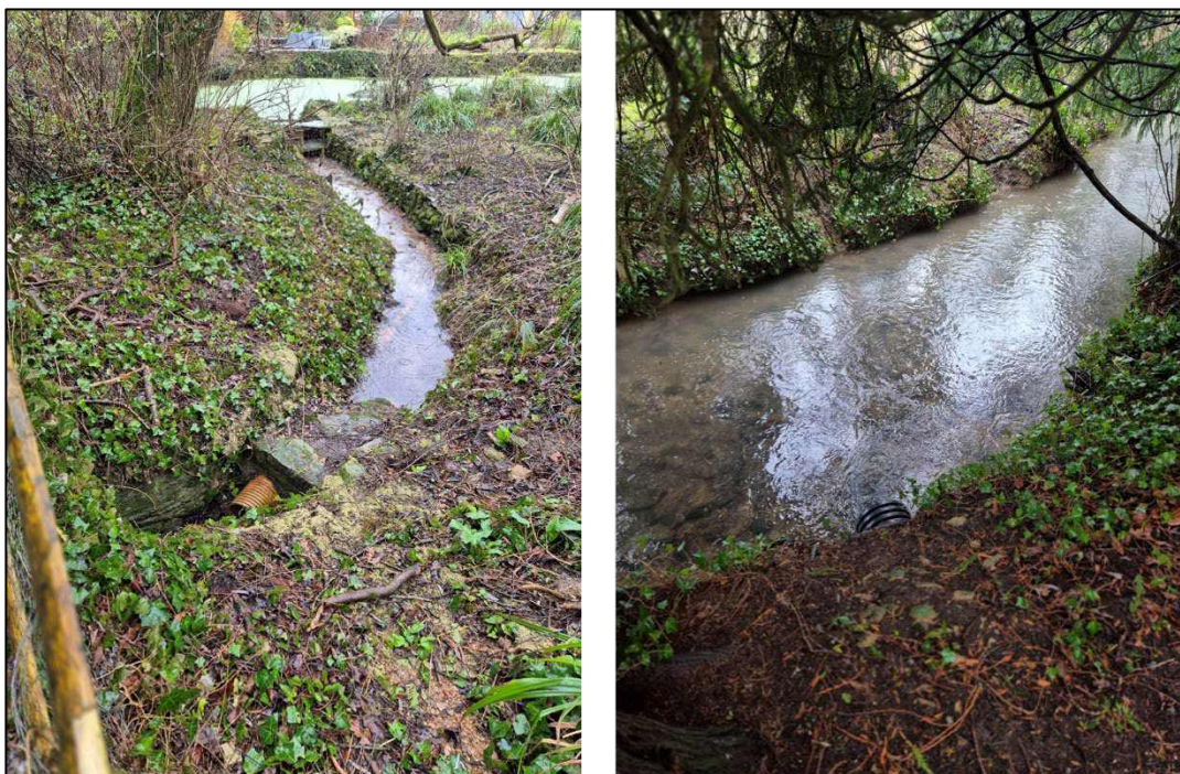
Figure 2-11 Flow controls and downstream pipework from Broughton Hall Pond
